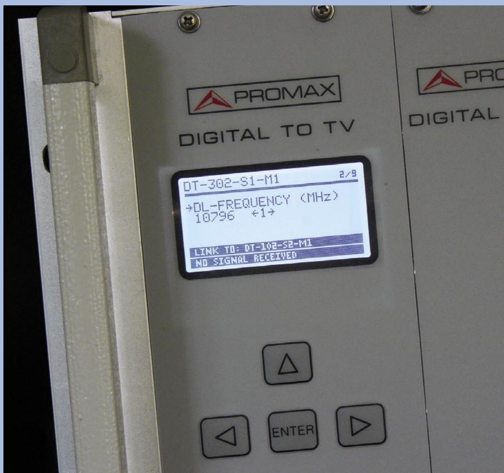
■ Setting up DT 302 module. You can see setting the frequency of the transponder to be received and demodulated to the pure transport stream.
